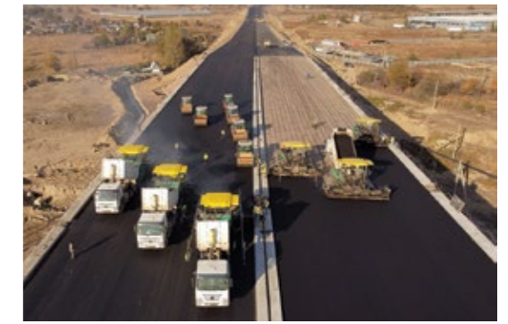
One of Kazakhstan's major public-private partnership project, it is designed as a 66 km long ring road through the Karasay and Talgar regions of the province of Almaty.
